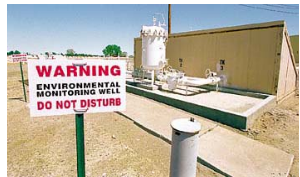
Testing stations to determine if there is a fuel spill dot the area of the underground fuel storage tanks at the Fallon Naval Air Station.
